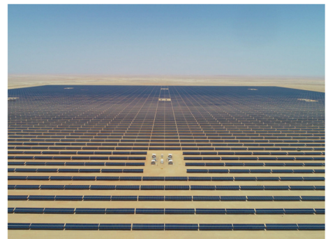
Sterling and Wilson Solar built this 125 MWp project in Oman Image: Sterling and Wilson Solar
