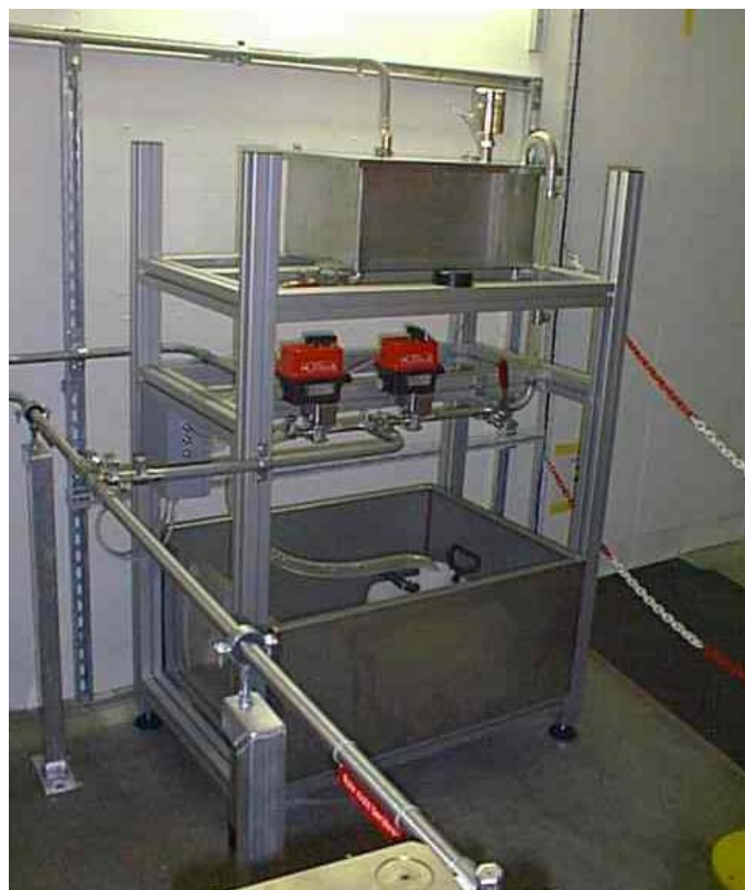
Fig. 8: Inner filling station. The two red pumps for draining (left) and refilling (right) of the HLS can be completely remote controlled. The inner filling station is directly connected to the half-filled HLS pipes which can be seen at the lower left corner of this figure.
