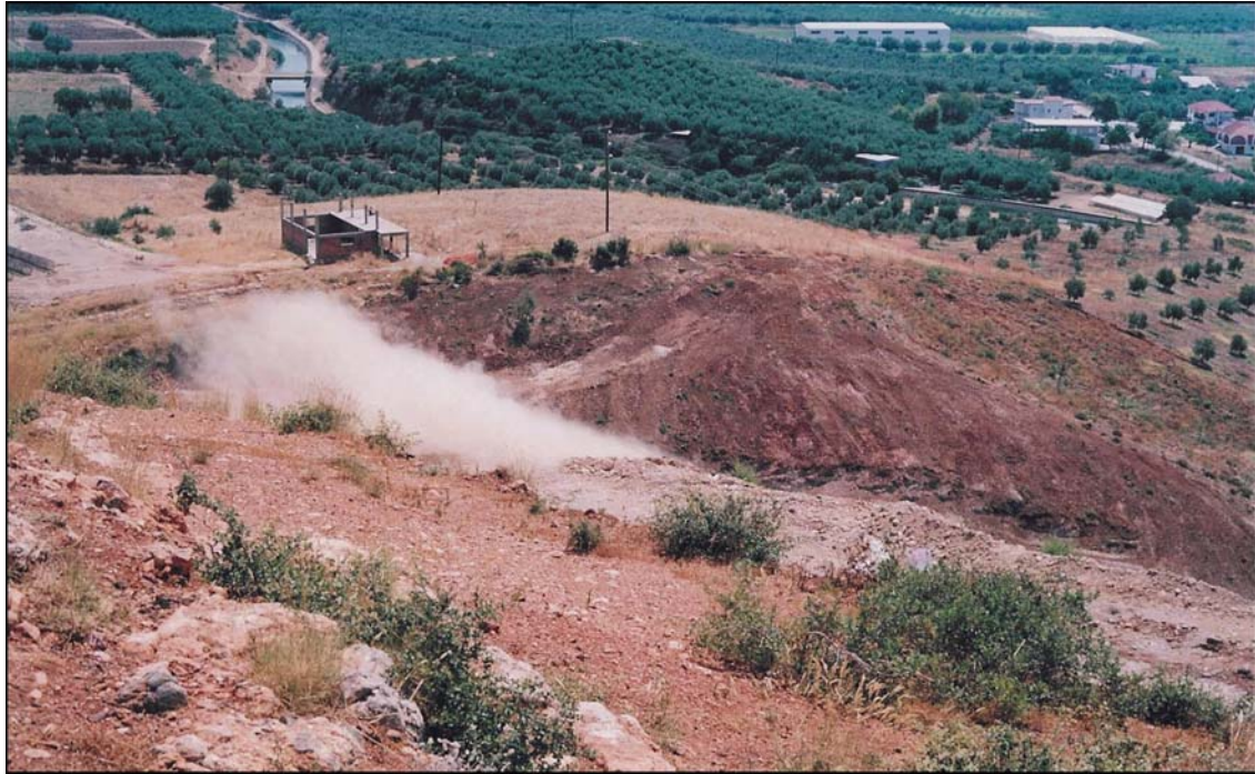
Photo 3: Blasting at 10 m. away from the ancient wall. Close and safe blasting may be possible!
